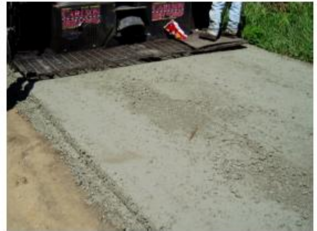
Figure 4.10 Segregation of RCC mixtures
