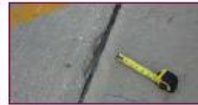
Spalling at cold joint
