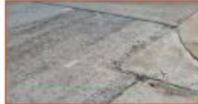
Mixture tends to segregate during paving and compacting
