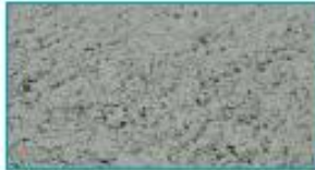
Mix too dry
