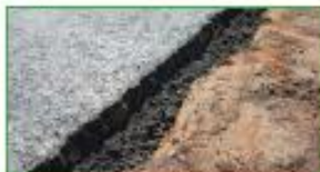
Edge slumping / poor consolidation at edge
