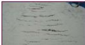
Minor tearing of the mix from rolling
