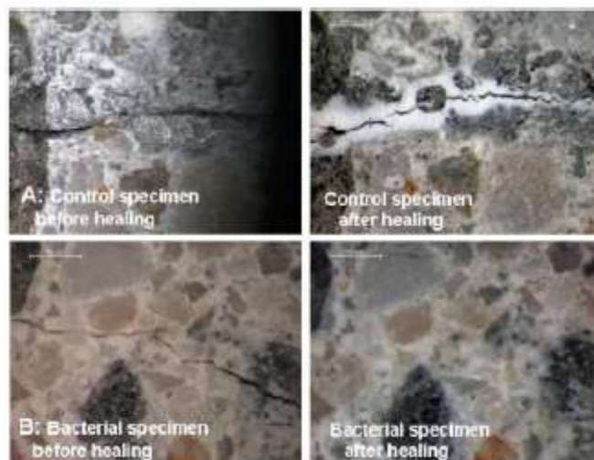
Figure 5. Cracked concrete specimens containing porous aggregates with food only (A) (top) and food plus bacteria (B) (bottom). The left figures are before and the right figures are after the healing.
