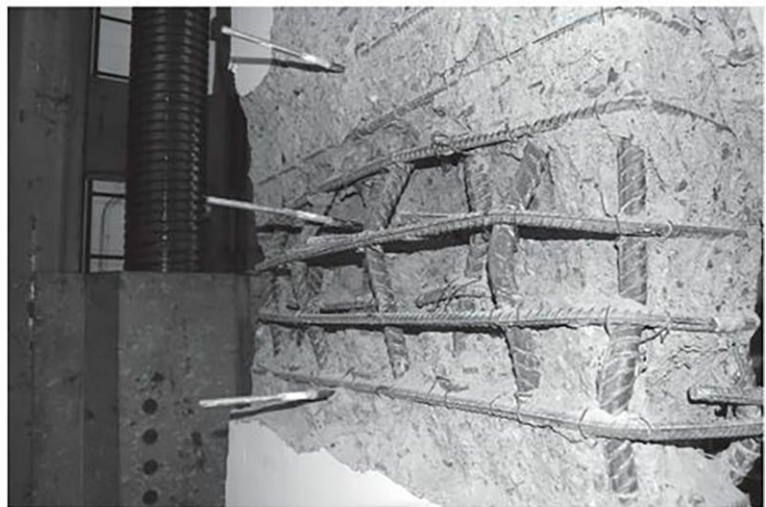
(c) Photograph of failed section
