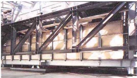
Fig. 4.11: Ice storage tank - Crystal Tower.
