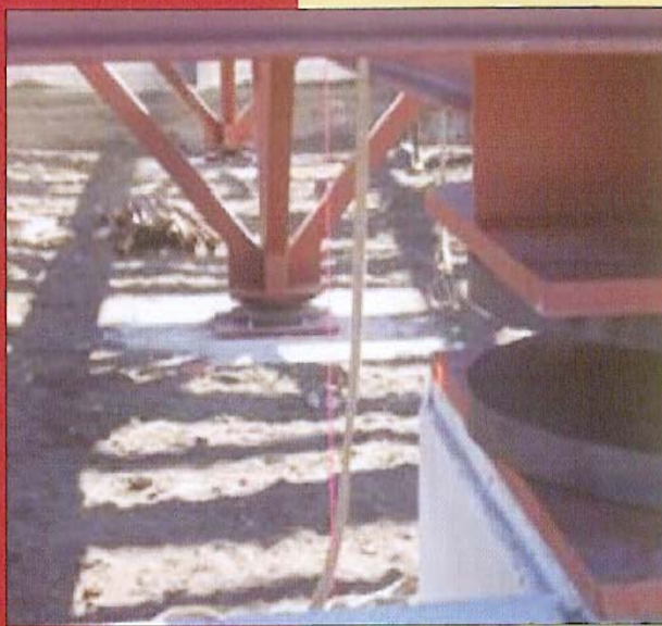
The new RoGlider™ being installed beneath the new Wanganui Hospital, Wanganui, New Zealand
